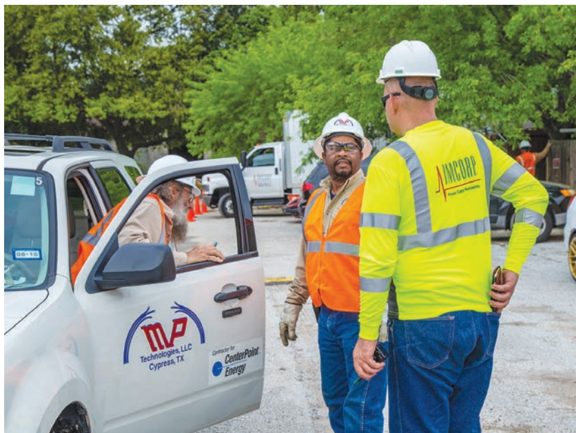
Teams of technicians work together to perform an assessment and complete any on-site mitigations, which includes isolating the cable and connecting the assessment equipment, performing the check and recording the results, and repairing or replacing terminations.
