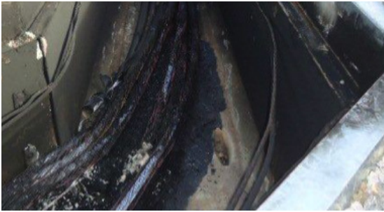
Cable damaged during installation and not detected with a VLF PD test.
