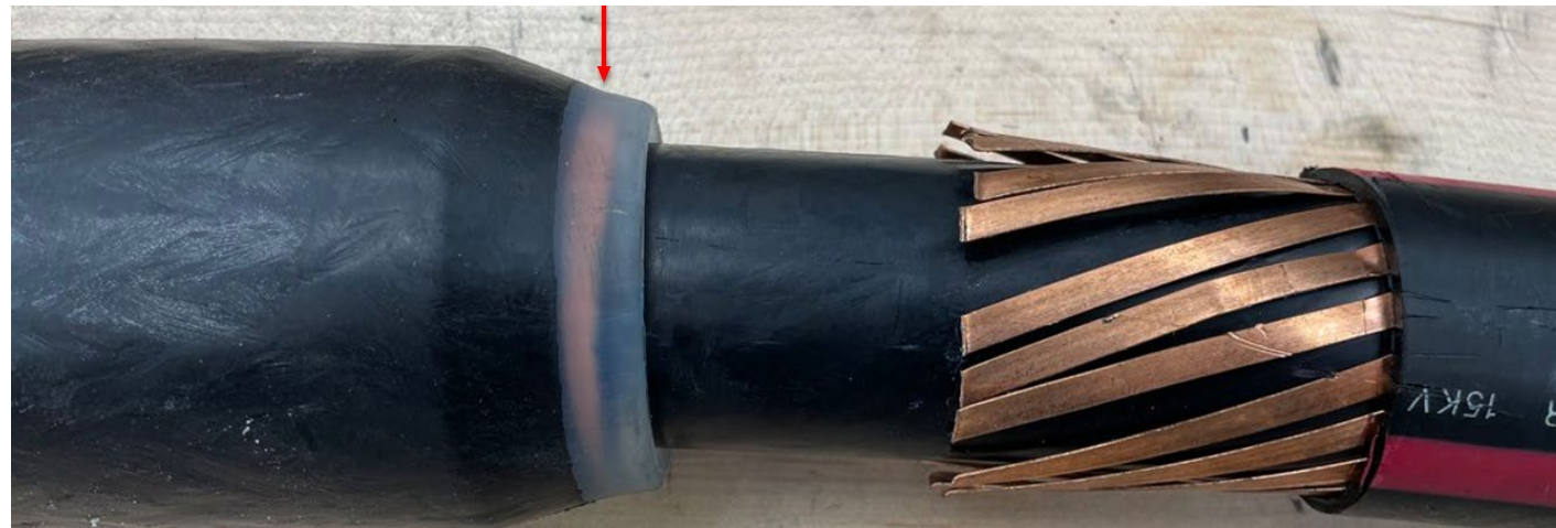
SPLICE BODY NOT OVERLAPPING SEMI-CON; INSULATION IS VISIBLE
