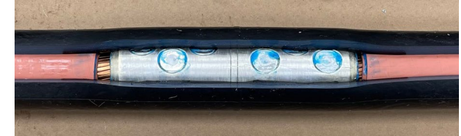
BLUE DISCHARGE CONTROL COMPOUND (DCC) SCARCE ALONG INSULATION
